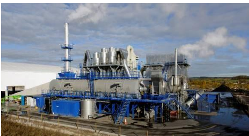
Figure 3. The thermal desorption plant.
